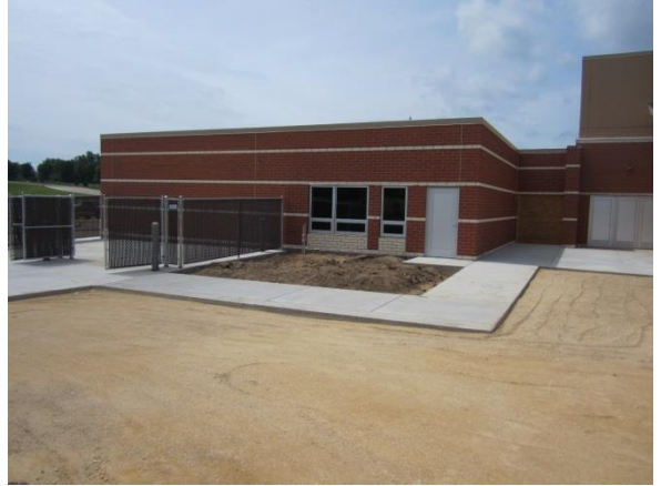
The exterior of east side is nearly complete as well. Paving took place on August 15 th .
