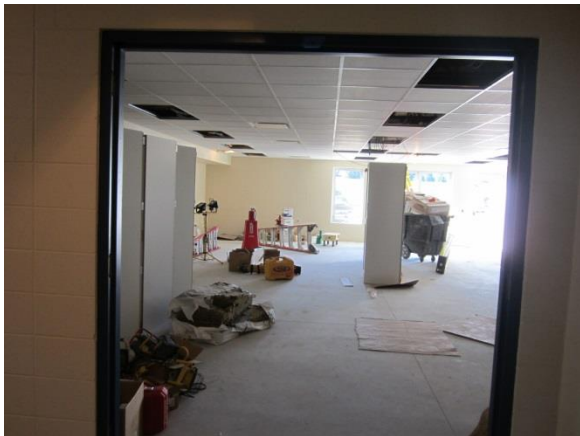
The classrooms are taking shape. Flooring will be the final item installed in the classrooms.
