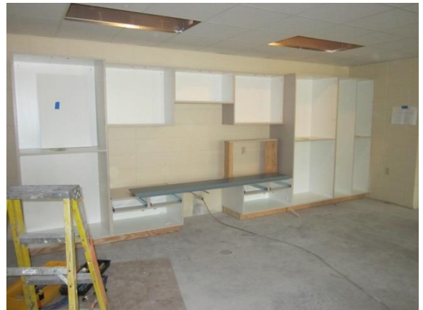
Carpenter's have been working to get the casework installed in the classrooms.
