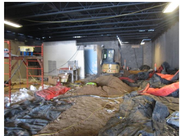
Plumbers have begun work on the underground piping to serve the new gym.
