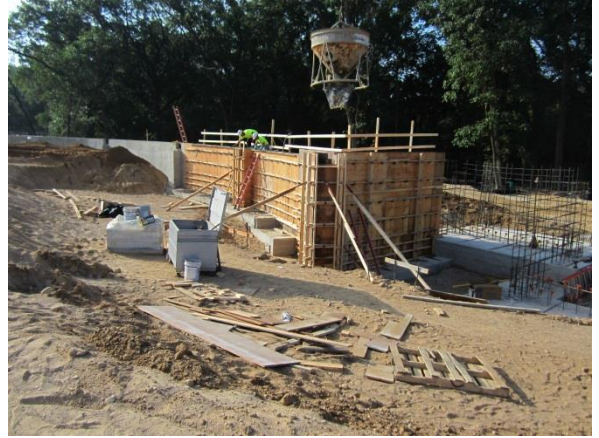
Concrete crews have been forming and pouring the radius foundation walls of the cafeteria.
