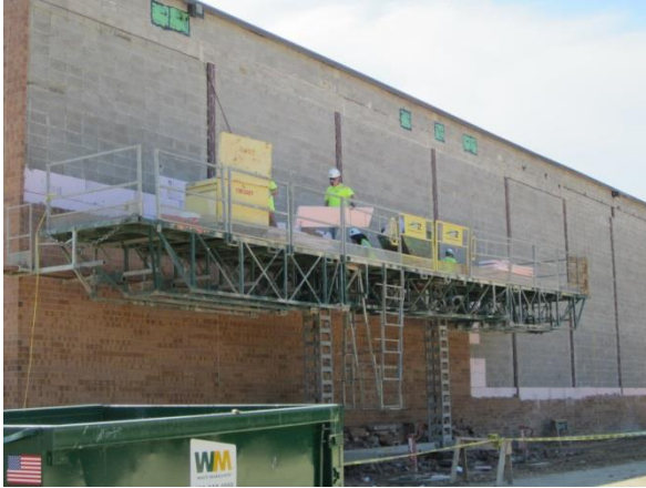
Masons remove the brick from the existing gym. The gym will remain and a new wall will be built next to it.
