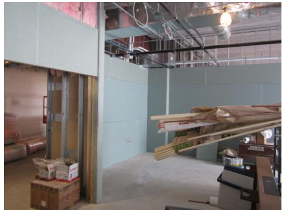
Drywall is on the walls in the 5 th grade classroom. In the next couple weeks the rooms will receive paint.
