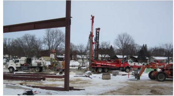
Geothermal well drilling continues in what will become the new parking lot.
