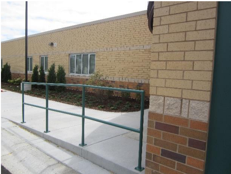
The safety railing was installed and painted at the exit out side of the Art Room and Careers Computer Lab, all vegetation has been planted- Site
