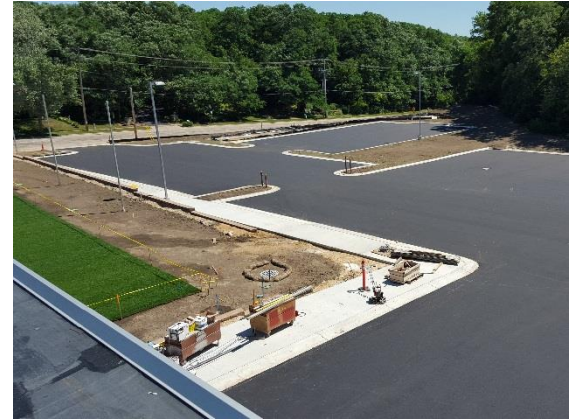
Asphalt Paving! Finally looking like a parking lot. Striping will be starting early next week!
