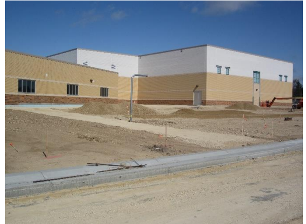
The east end of the site is ready for the pouring of sidewalks
