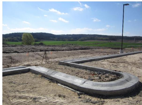
Concrete curb has been poured at the east end of the site
