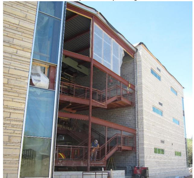
Structure for the 6 th , 7 th and 8 th grade stairs is being installed – Area A
