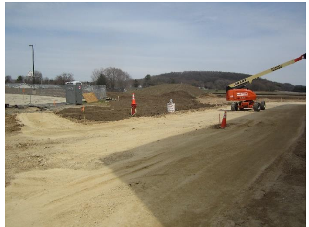
The Findorff job trailer has been taken off the site; the field office has moved to the new art room
