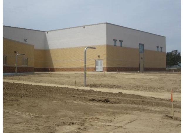
Poles for exterior basketball hoops and gravel base for sidewalks are in place - Site
