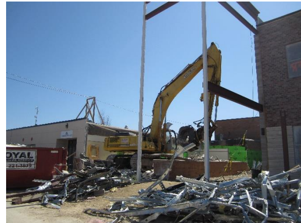
Existing administration offices have been demolished in preparation for the completion of the 5 th grade wing
