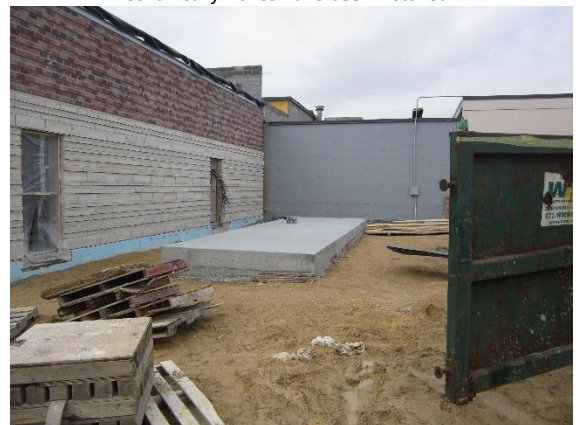
The emergency generator pad has been poured in preparation for the arrival of the generator
