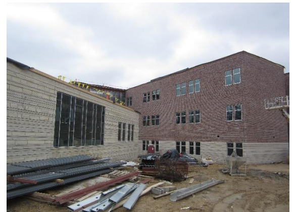
Windows and curtain walls are in place in area C. Area B windows are being installed.
