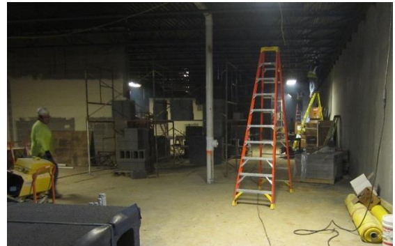
The slab on grade has been poured in the locker room and block walls are underway.
