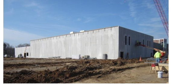
All of the precast wall panels have been set and opening are being cut into the panels for the windows.
