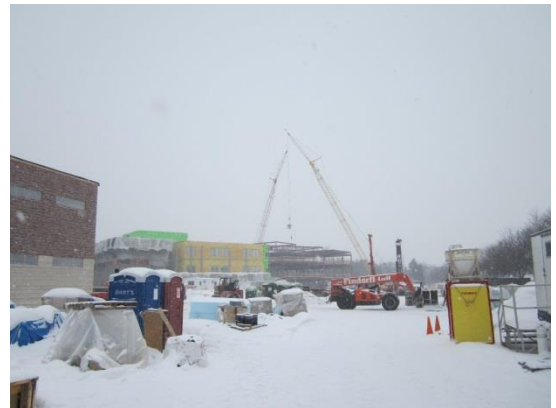
Work continues through the snow onsite. The final pieces of structural steel were set this past week.
