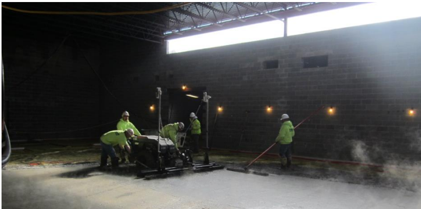
Workers use a laser screed to strike off and level a concrete slab.
