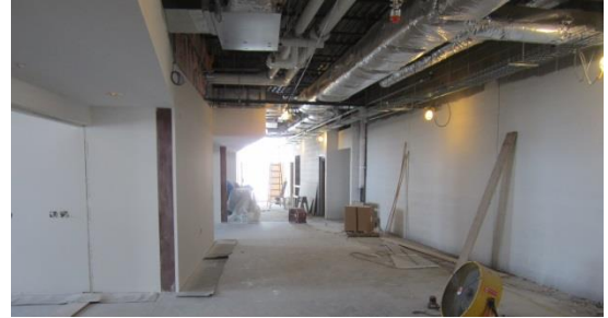
Drywall is up in the 5 th grade wing and painting has begun.
