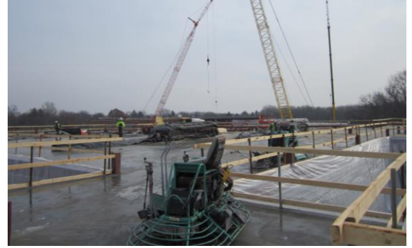
Workers remove blankets from the concrete slab on the 3 rd floor near the library.
