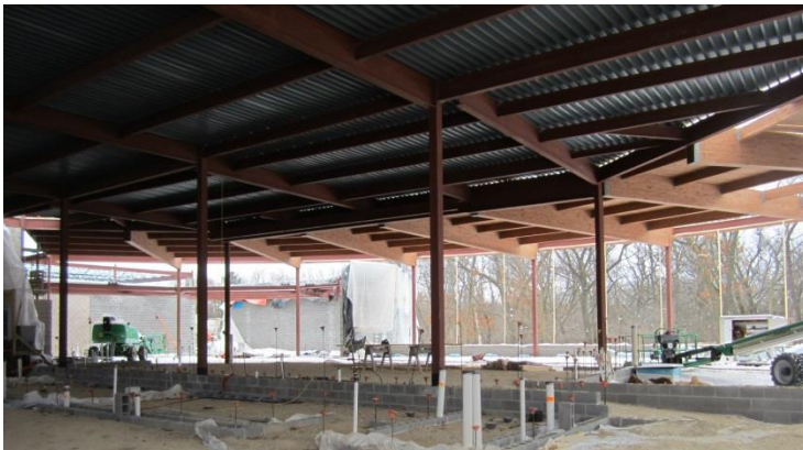
The glue laminated timbers are up in the cafeteria and ready for a roof.
