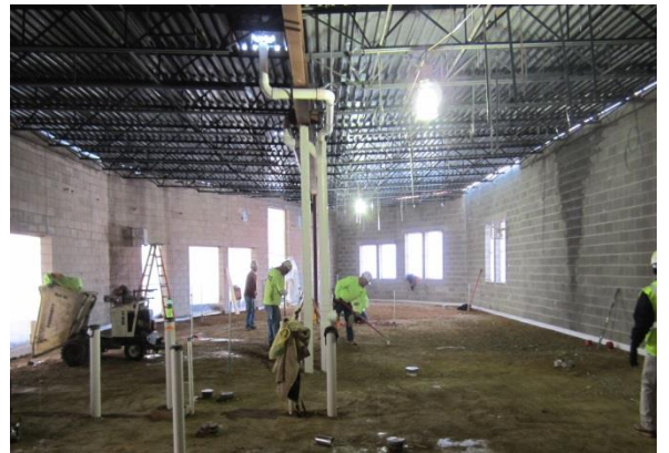
Workers prepare for the concrete slab on grade in the student services.
