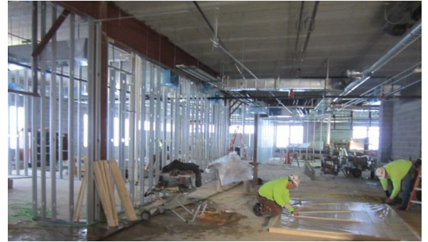
Steel studs are up in area D and the MEP subcontractors have begun in wall rough-ins.
