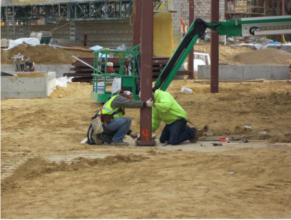
Ironworkers set a steel column for the frame of the 6 th , 7 th & 8 th grade wing.
