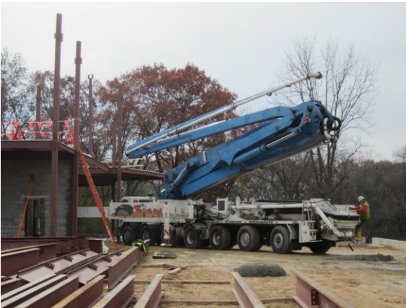
In order to get concrete to the 2 nd floor of the building a concrete pump truck is used. This particular truck is able to pump concrete 200' in the air.
