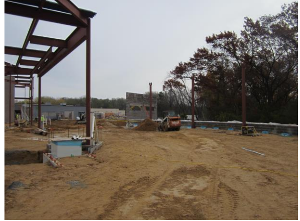
Work is progressing in the cafeteria. Next week the timbers will arrive to form the roof.
