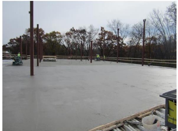
The first concrete slab for the 2 nd story was poured on Friday. The area pictured will be the new Library.
