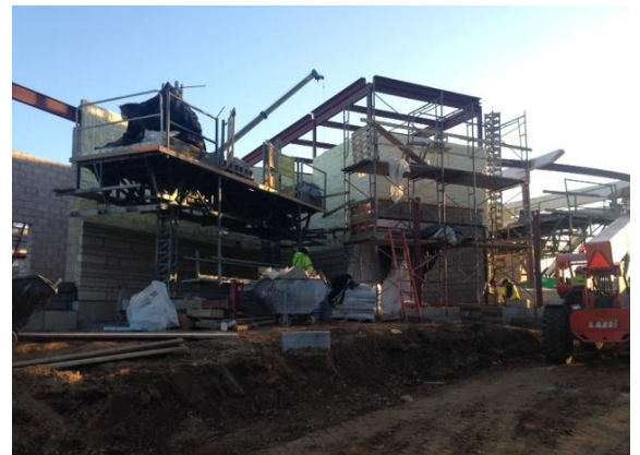
Crews are working on installing the stone veneer on the exterior of the building near the conservancy.
