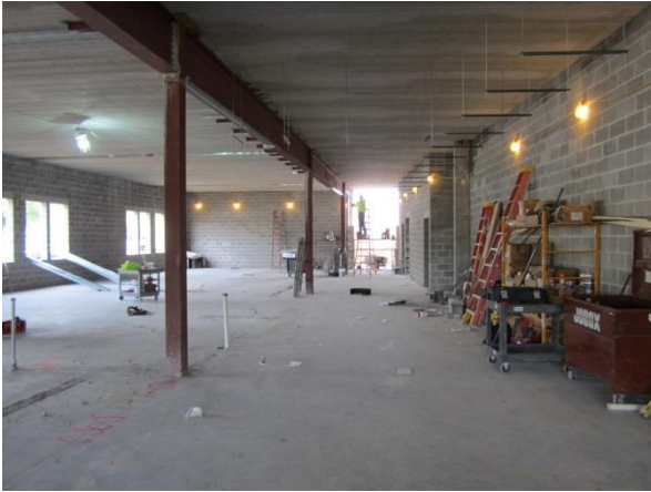
Inside the 5 th grade wing mechanical, electrical, and plumbing rough-ins have started.
