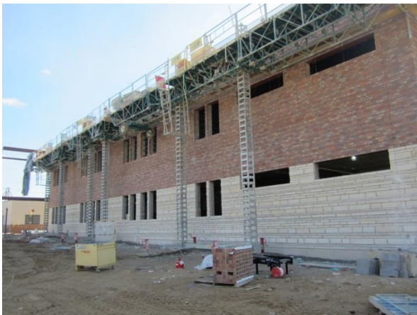
Along Donna Drive the installation of the brick and stone facade of the 5 th grade wing is underway.
