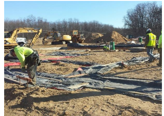
Concrete footings have been blanketed to protect them from the cold weather.
