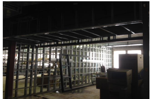
Wall framing is complete in the 5 th grade wing and subcontractors are installing mechanical and electrical systems in the walls.
