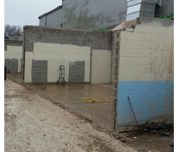
Selective demolition is complete in the locker rooms. The walls shown above will remain for the new locker rooms.
