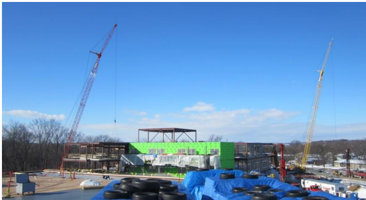
Looking west from the existing gym the new school continues to take shape.
