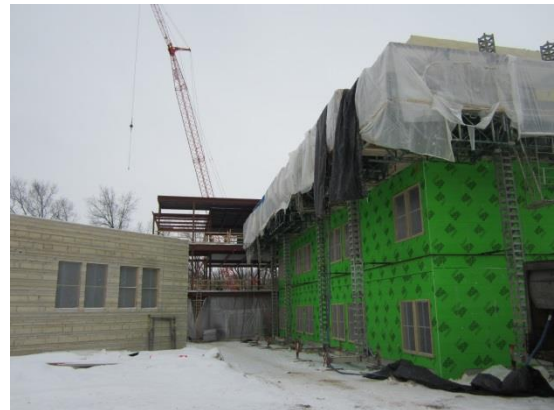
Sheathing is on the exterior walls and spray foam insulation is being applied in preparation for brick and stone.
