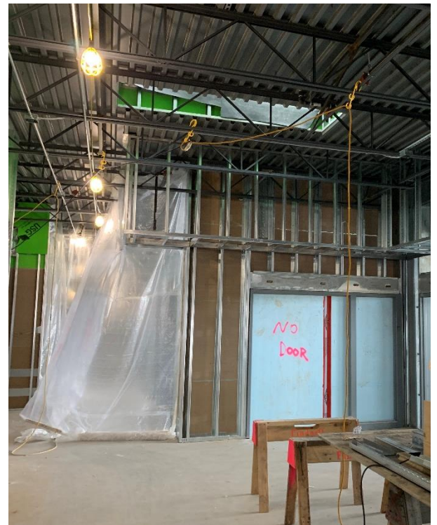
Above: Temporary partitions to contain the heat in portions of the building.
