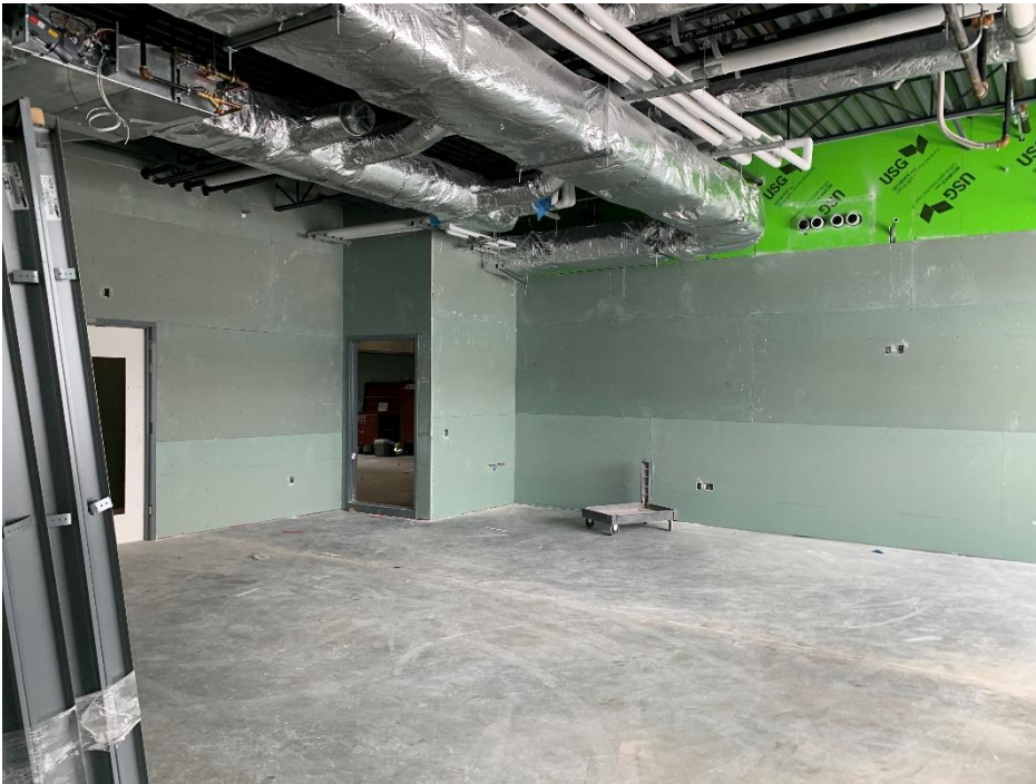
Above: Fully drywalled first grade classroom with insulated HVAC ducts. The walls are ready to be taped and painted.
