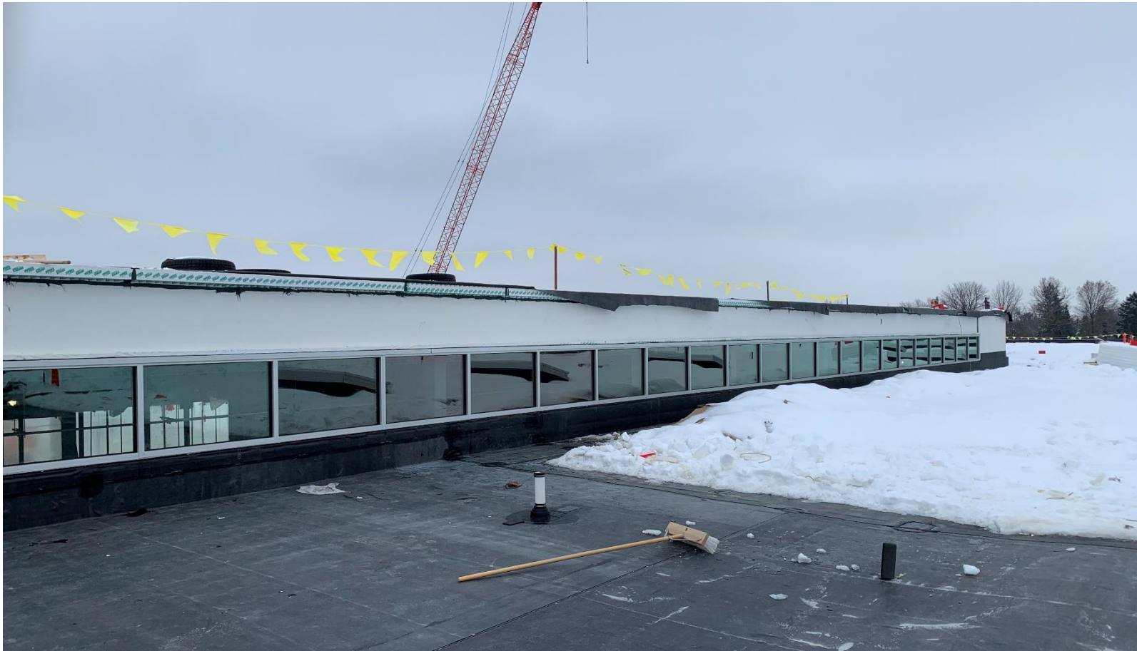
Above: Clerestory windows have been installed along the roof. These windows now allow natural light to filter down into the school.
