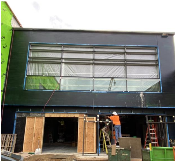
Storefront window frames installed on the second floor in the concourse vestibule. Glass beginning installment.
