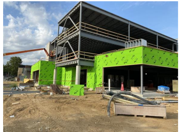
Exterior studs and sheathing installed on the outside of the east side of the north addition.
