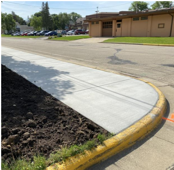
New concrete sidewalk poured on south side of existing school along Park Street.
