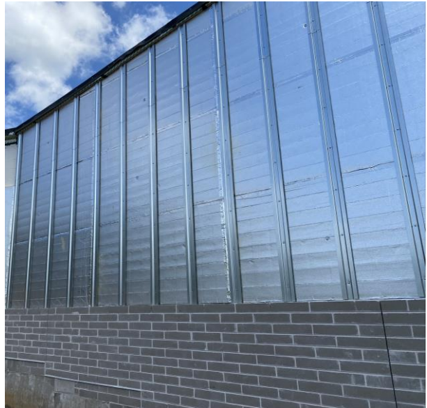
Hat channel installed on exterior of addition in preparation for metal panels.
