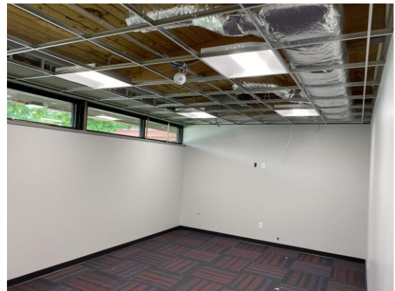
Carpeting, painting, and drop ceiling installed in new offices and conference room.
