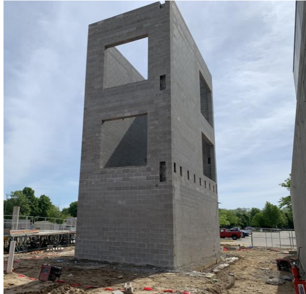
Stair 4 is now complete on the east side of the new addition.
