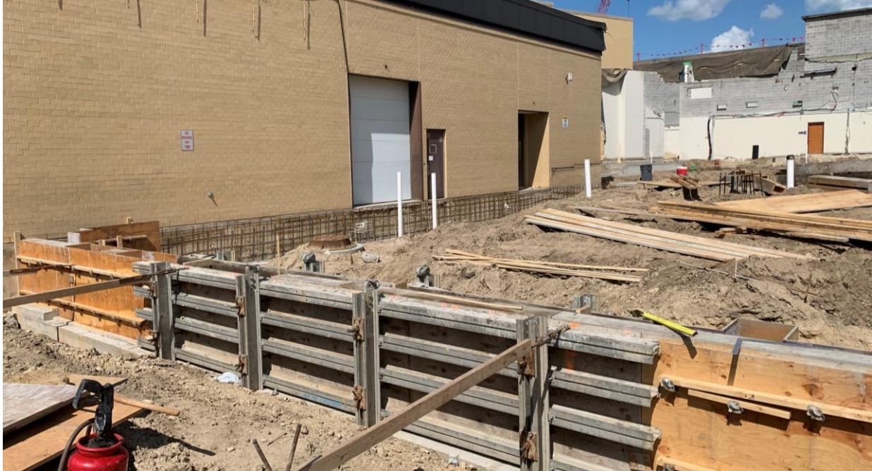
Concrete forms set on the footings and foundation walls poured in the Black Box area.
