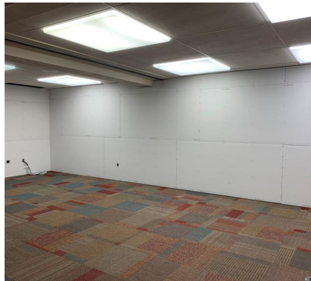
Drywall set on the interior studs in the LMC for the temporary classrooms.
