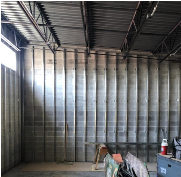
Steel stud framing added to cafeteria in preparation for drywall to be hung.
