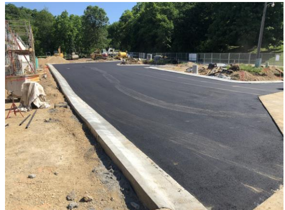
Curb and Gutter poured and binder course of asphalt laid in the new parking lot extension.
