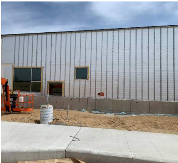
Furring for metal panel installation have been placed on the west side of the building.
