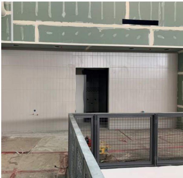
A grey tile backsplash has been installed outside of the 2 nd floor atrium bathrooms.
