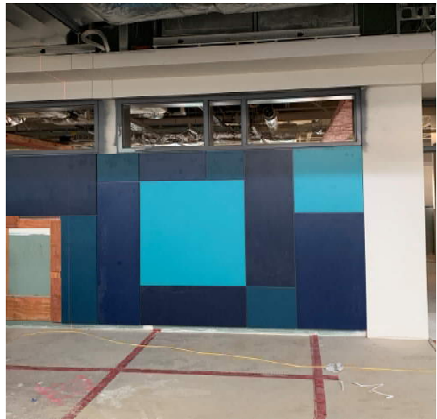
Blue interior wall panels have been installed in the cafeteria area of the atrium.
