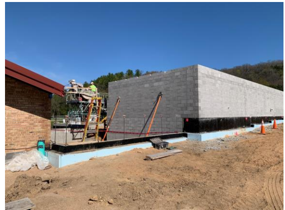
View looking to the north. CMU erected on the south and east walls of the new kitchen.
