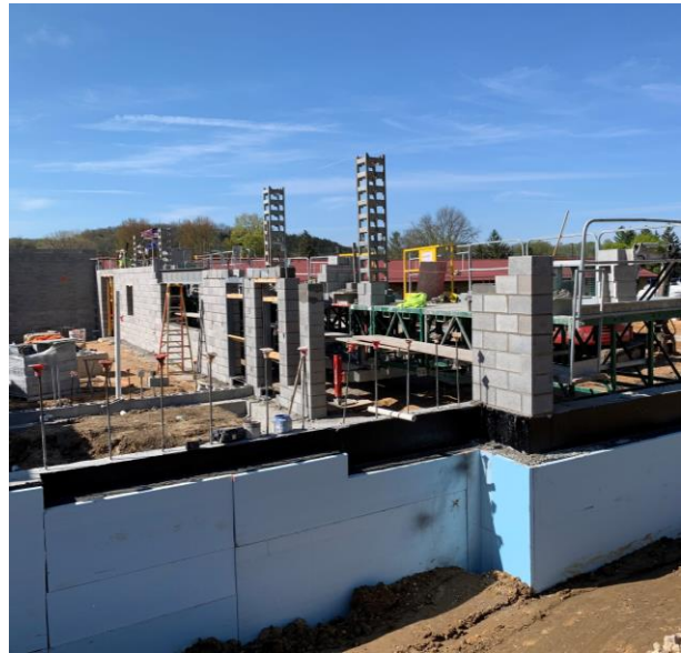
The middle loadbearing wall under construction. Also visible is the waterproofing and insulation applied to the foundation walls.
