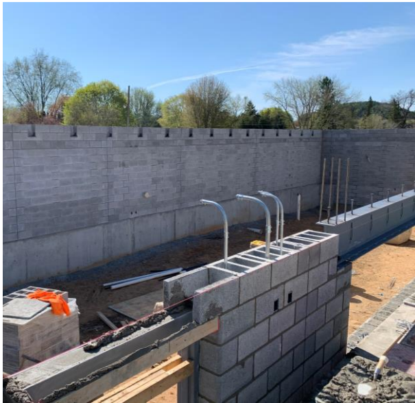
View of the eastern CMU wall. Grout and more CMU is being laid on the middle wall.
