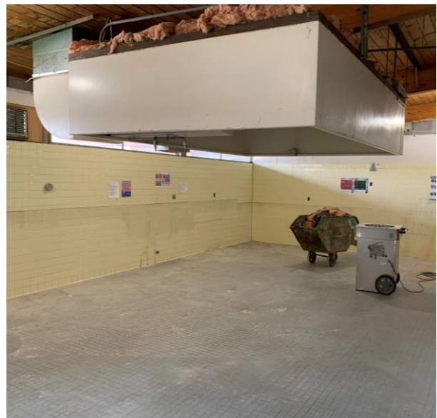
The former kitchen has been cleared of equipment and demo has begun on the louvers and walls.
