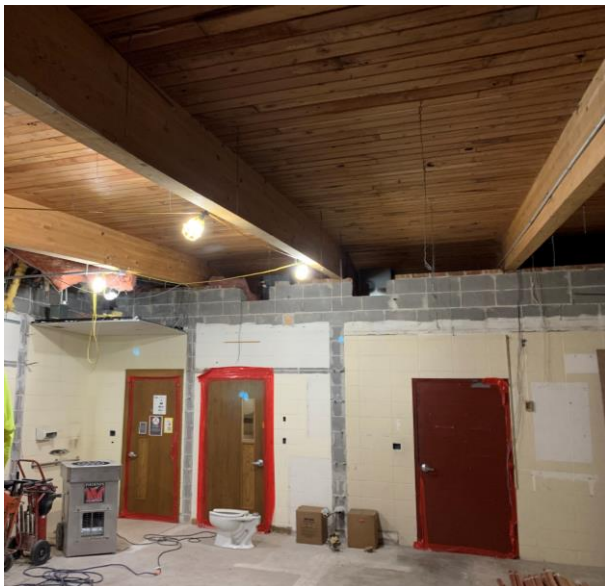
Demo in the guidance room, custodial office, and small bathroom to remove the walls, flooring and ceiling.
