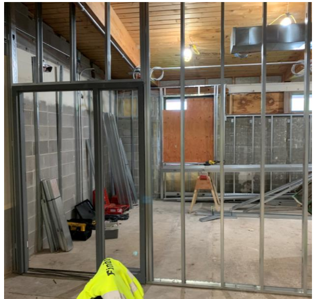
Steel studs and doorway set for the new conference room and offices.
