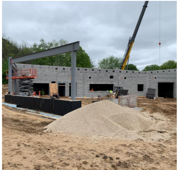
Steel columns and beams set on the north side of the addition.
