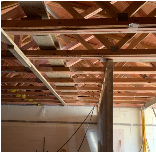
Wood trusses above the corridor to new cafeteria. More trusses were added next to the old trusses to allow the roof to carry more weight.
