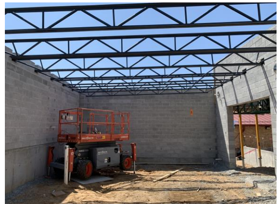
Steel trusses set over the bathroom and kitchen areas of the new addition.
