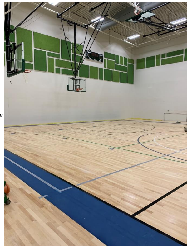
Right: The gym floor has been sanded; it is now undergoing painting and sealing.
