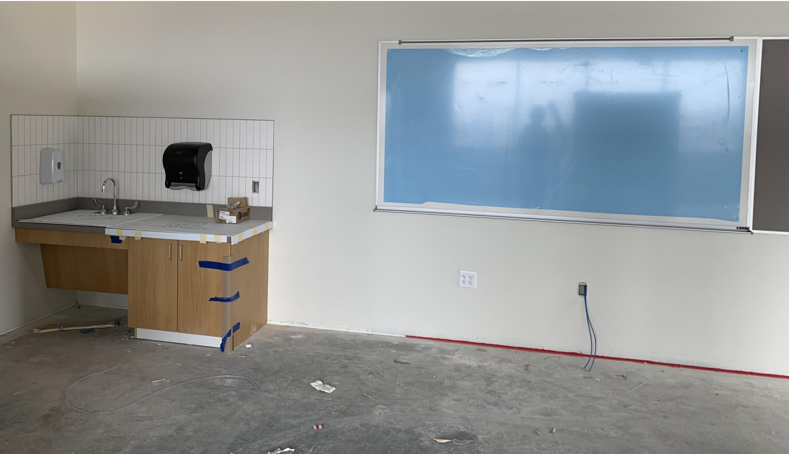
Above: A first grade classroom with a marker board and tack board installed on the wall. The sink has been installed in the cabinet, while the paper towel and soap dispensers have been hung on the tile.
