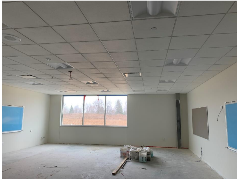
Above: Ceiling tile added to a second floor classroom. Lights and HVAC diffusers have been installed in the ceiling grid as well.
