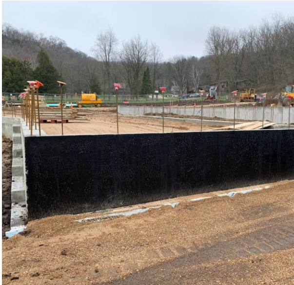
Water proofing efforts beginning. The black layer will help to prevent water from seeping through the concrete.
