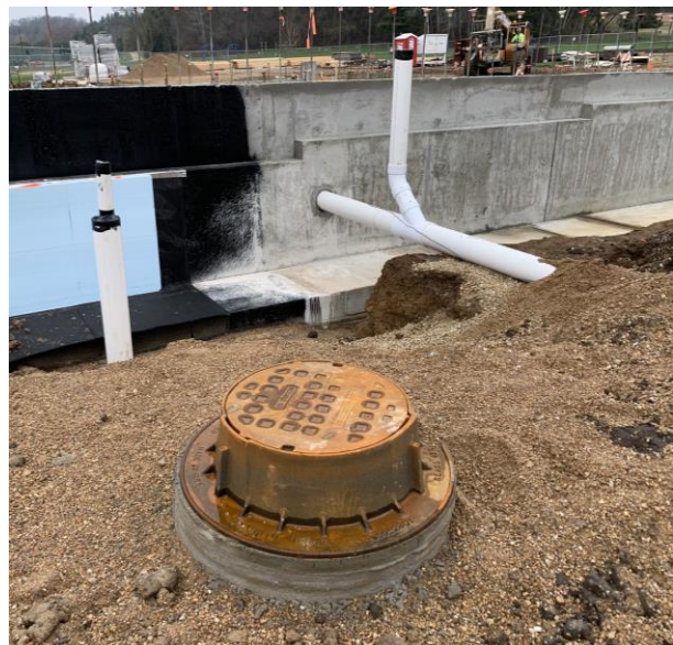
Storm line running out of the building foundation walls. This will allow rain water from the roof to be transported outside of the building's footprint.
