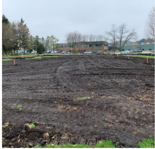
Field on the west side of the building has been filled back in and pitched correctly.
