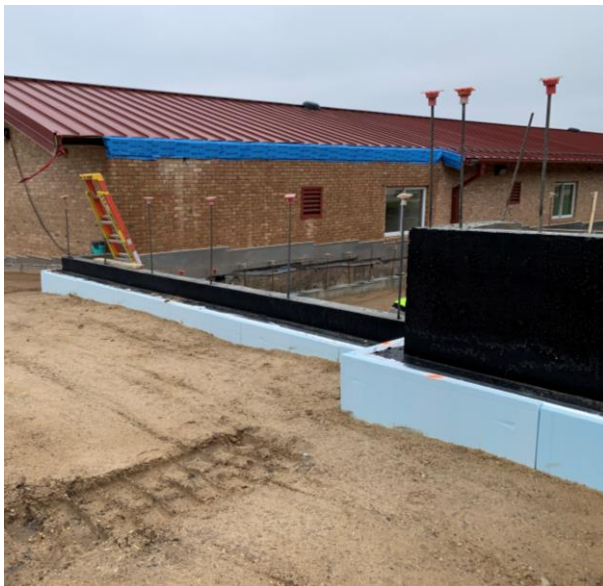
Insulation added over the waterproofing layer. This wall has been backfilled bringing the ground back up, closer to the top of the wall.
