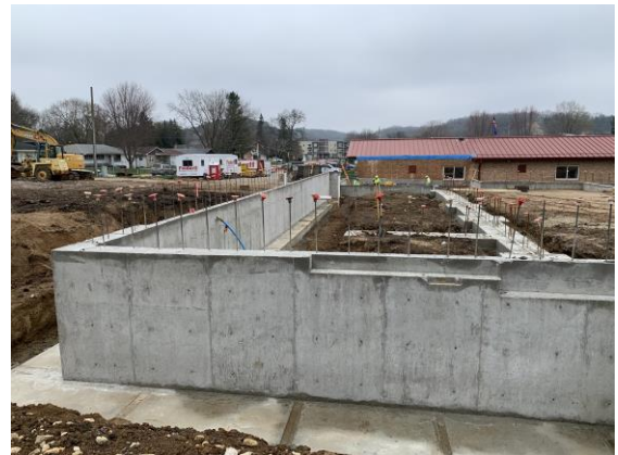
The north wall and the middle, load bearing wall have been poured and cured.
