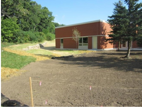
Landscaping is nearly complete on the west side of the school. With the cooler weather next week crews will be able to install the sod at the playground.
