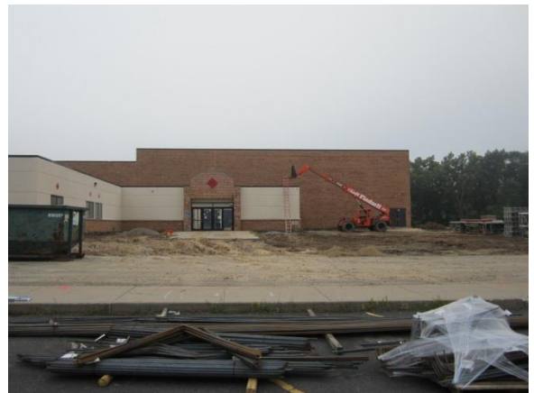
The main entrance has been removed to allow the construction of the 5 th grade wing.
