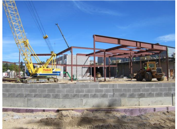
Looking north from Pheasant Branch, the structure of the cafeteria is beginning to take shape.
