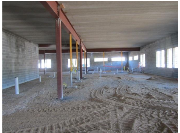
With the arrival of the precast floor planks the 5 th grade wing is partially enclosed. In less than one year classes will be underway in this space.
