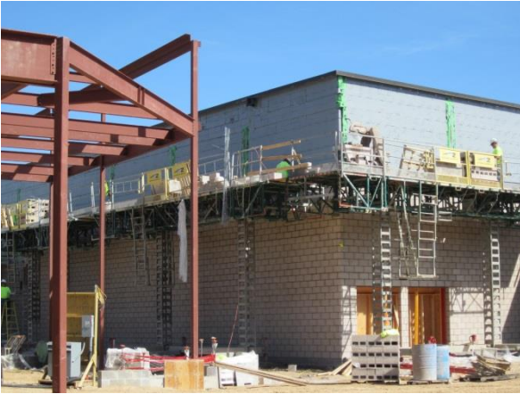
Burnished Block has arrived and is being installed along the existing gym.
