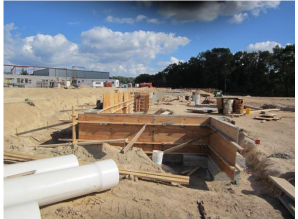
The foundation of the building is progressing east into the 7 th & 8 th grade wings
