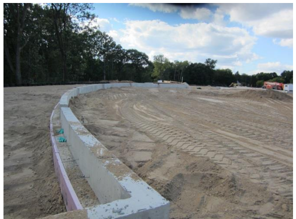
The radius wall of the cafeteria is now backfilled. When complete a glass wall will provide an expansive view of Pheasant Branch.
