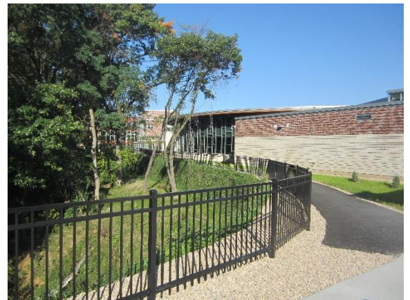
Completion of guard rails on the south side of the building - Site
