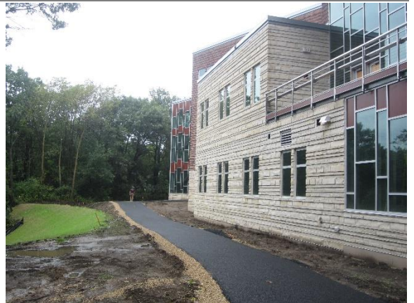
Porous asphalt at the path behind the 6 th , 7 th and 8 th grade wing is installed - Site
