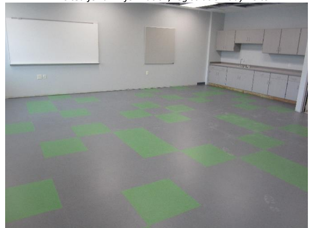
Vinyl floors are being installed in the 7 th grade classrooms. Carpet installation in the corridors is soon to follow – Area B
