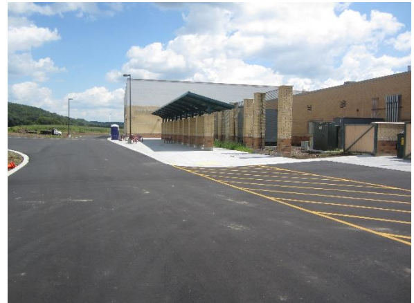
Asphalt top coat and striping are complete in all areas excluding the main lot - Site
