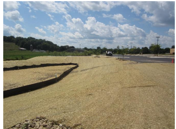
Seeding at the bioretention pond and front entrance is in place - Site
