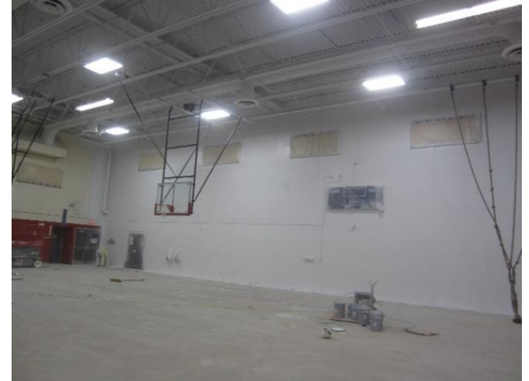
The roof deck and walls of the existing gym have been painted. The floor is being prepared for synthetic floor installation – Area D
