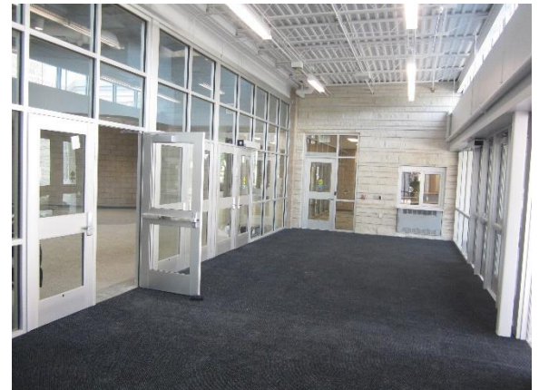
The main entrance vestibule has been painted and carpet has been installed – Area C
