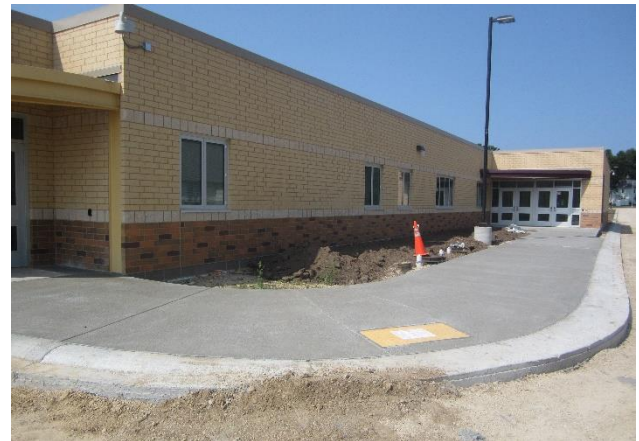
Concrete sidewalks have been poured at the entrance to the art and music room addition – Site/Area D
