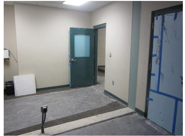
The wall dividing the existing band practice rooms has been demolished. The new room is ready for wall patching. – Area D
