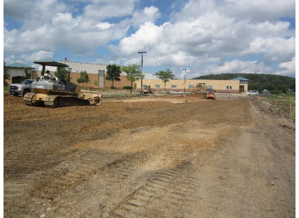
The main parking lot is being re-graded in preparation for curb, sidewalk, and asphalt installation – Site
