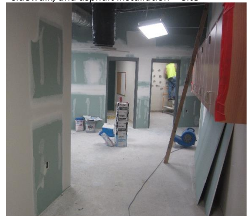
Drywall has been installed and taped in the student services area. – Area C
