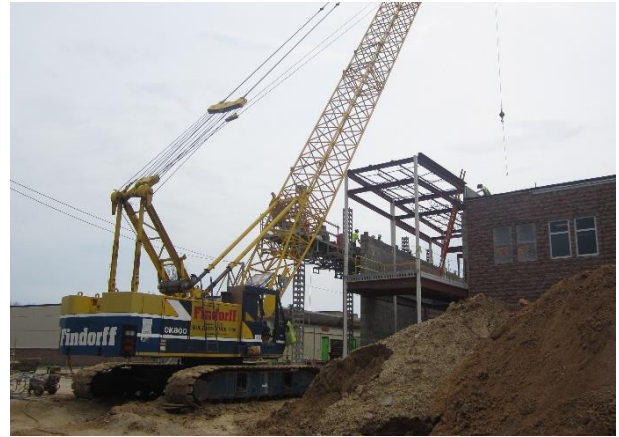
Roof joists for the 5 th grade stairwell are in place and masonry walls are being constructed – Area D
