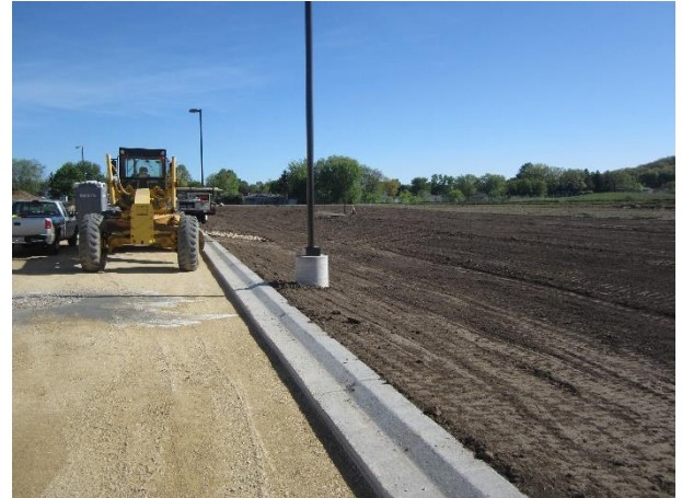
Top soil is being placed at the east end of the site.
