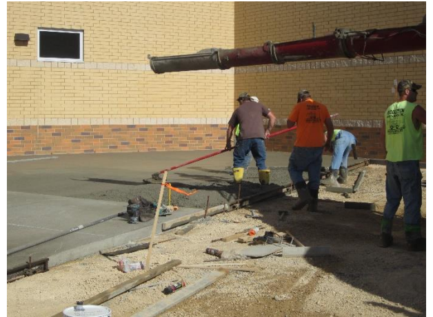
Concrete crews continue to work around the east end of the building.
