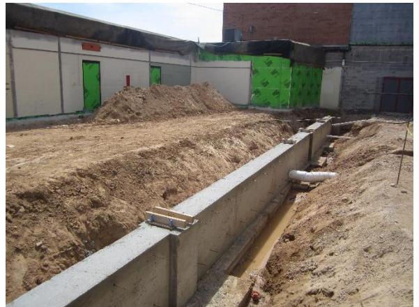
Footings and frost walls for the 5 th grade wing have been poured – Area D
