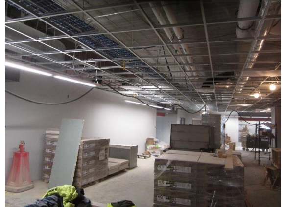
Area D casework has arrived, and lighting fixtures and mechanical finishes have been installed
