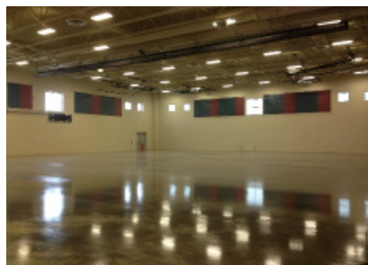
Gym Floor Moisture Mitigation – Area F
